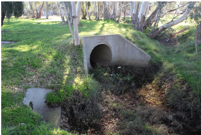
Figure 2- Poorly designed stormwater outlet
