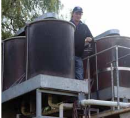
The mixing tanks
