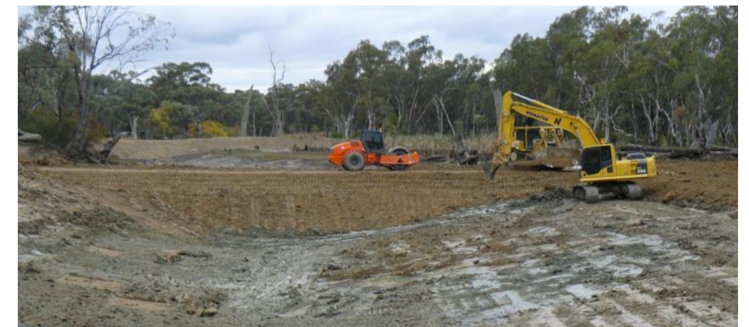
Work has commenced preparing Gunbower Creek for the construction of the new Hipwell Road Weir. Photo: Anna Chatfield.
