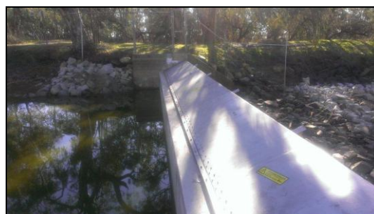
Figure 6: Concrete reinforcement of the Quambatook Weir commenced in May with the gate fitted in June 2013 (Photo: Gannawarra Shire Council)
