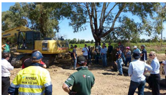
The Cohuna farm walk looked at the installation phase of an irrigation modernisation project
