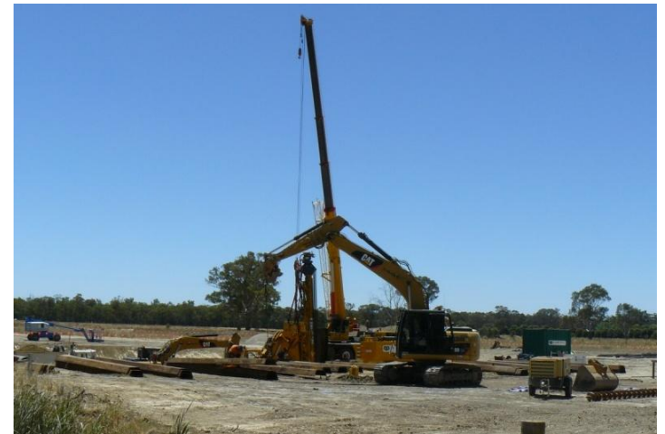
Work starts on the Offtake Regulator at Hipwell Road. Photo: A. Chatfield
