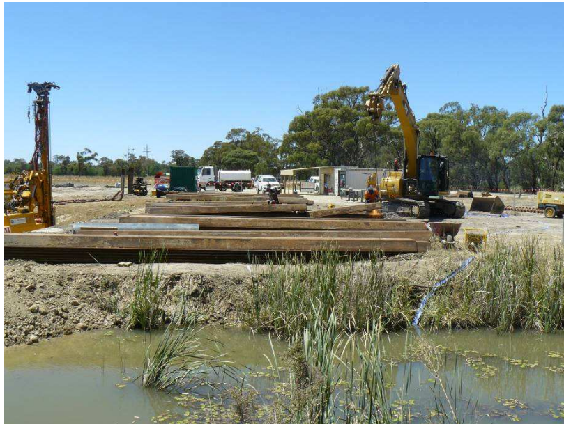
Photo 1: Steel sheet piles ready to be installed as part of the Offtake Regulator.
