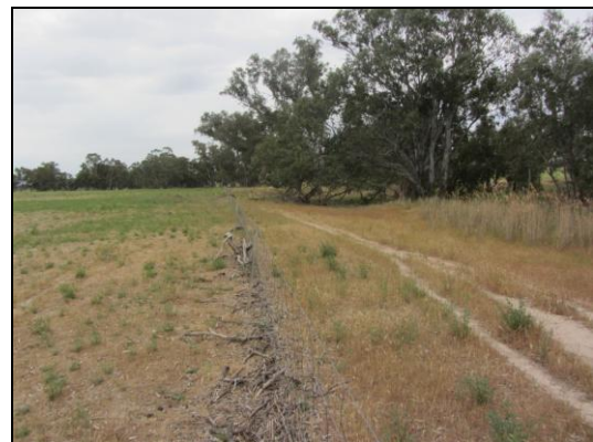
Figure 2: Before works - flood damaged fence along Avoca River at Archdale
