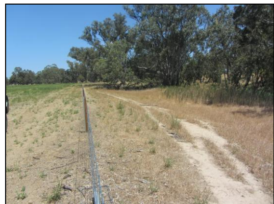
Figure 3: After works - more resilient 'lay down' flood fencing reinstalled to protect the river frontage
