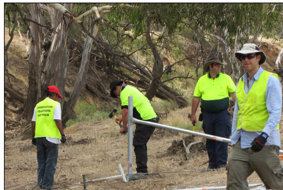
Figure 1: CVA crew replacing flood damaged fencing along the Campaspe River, Rochester. Photo: North Central CMA
