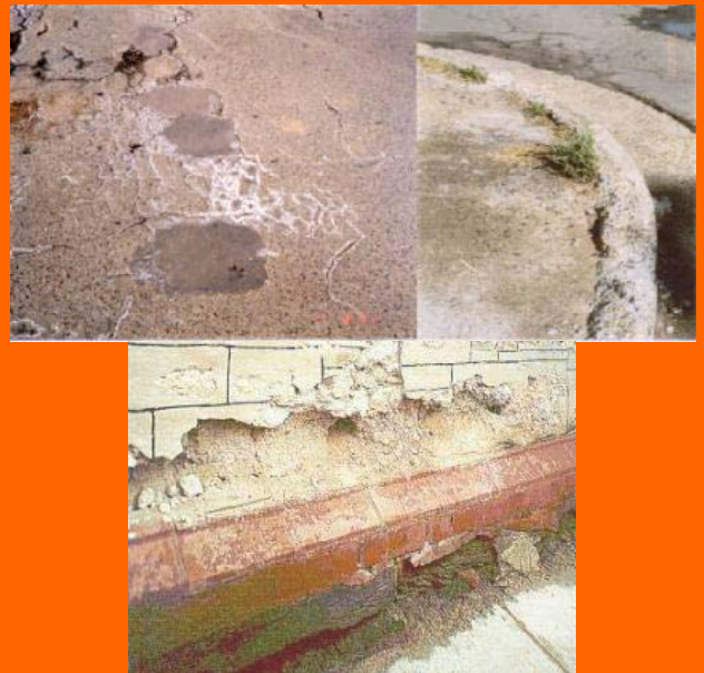
Examples of salt damaged infrastructure
