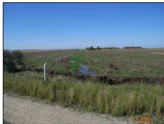
Regional drain requiring silt removal. Photo: North Central CMA
